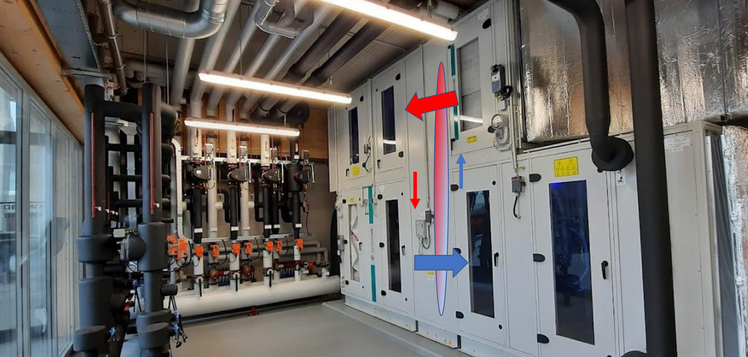
The warm air from inside the building heats up the refreshing cold air from outside. This saves 80% energy.
